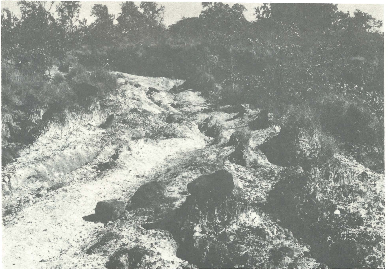
Figure 22. Soil and rock erosion of an old road on white volcanic ash soils where oak forest once stood in interior Hacienda Poco Sol.
